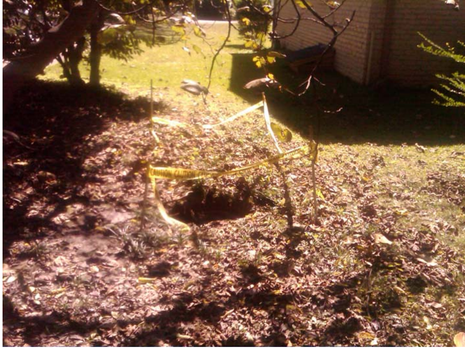
Photo 3 -- Collapsed section of pipe; box top has caved in.
