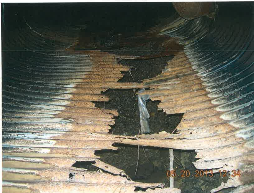
View of existing pipe invert showing extensive rusting and deterioration; subgrade soil is eroding.
