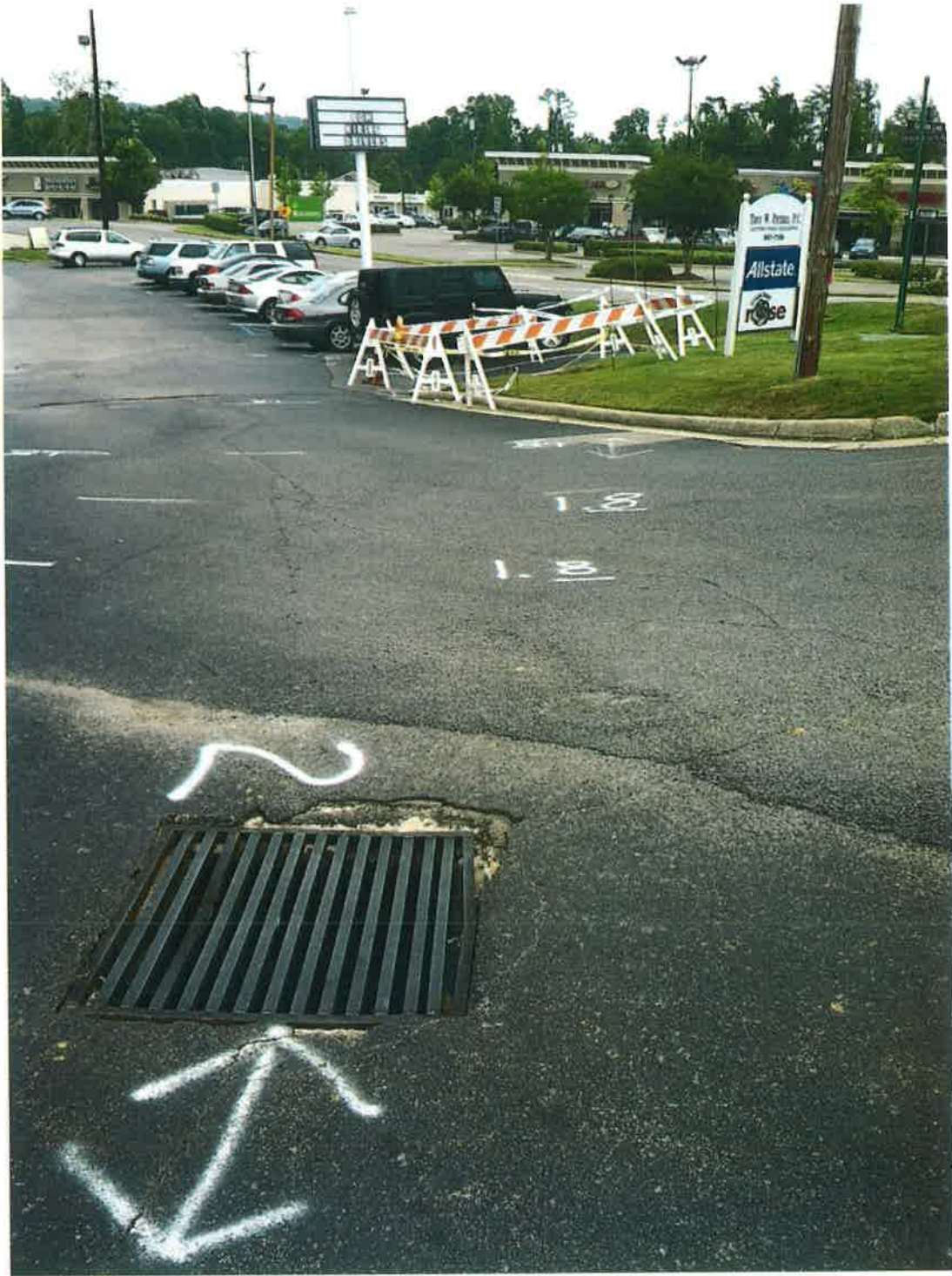
Looking downstream at route of deteriorated drainage pipe; this is at asphalt drive and parking area at 4200 Oakview Lane (Peters) looking down to corner parking space at 3135 Cahaba Heights Road (Cahaba Heights Plaza) and Cahaba Heights Road right-of-way.
