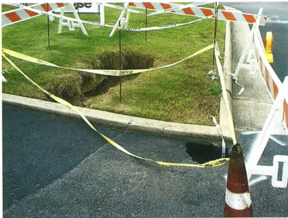
Area of collapsed asphalt and median area at parking area for Cahaba Heights Plaza; metal drainage pipe has deteriorated allowing dirt and subgrade to be eroded out from under and around pipe.
