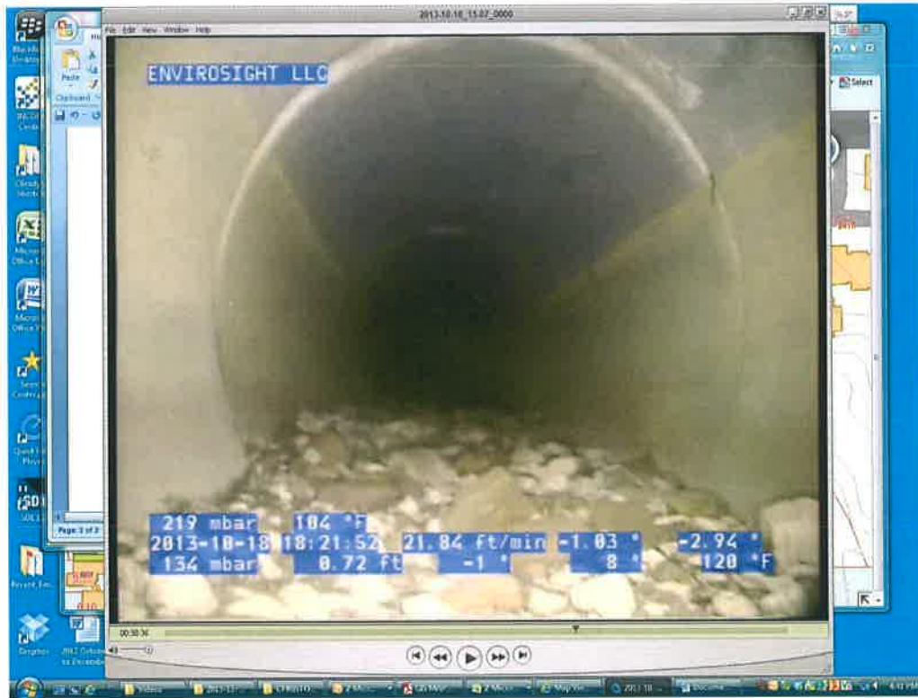
Photo 4: debris in pipe, 24" RCP
