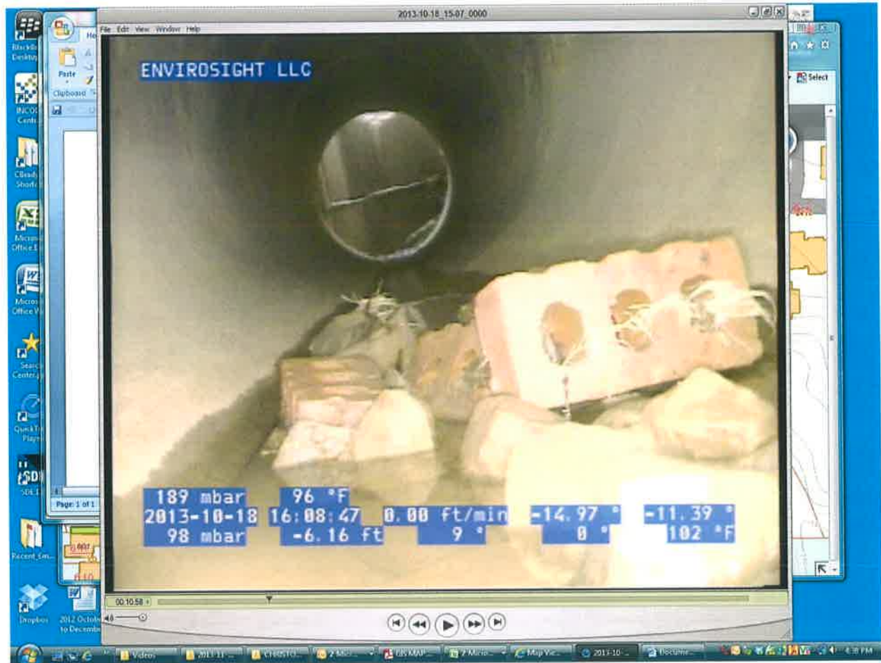
Photo 1: debris in pipe, 24" RCP,
