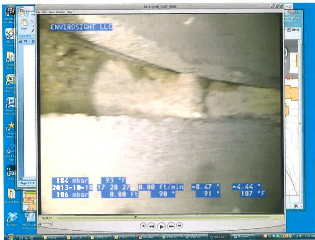
Photo 2 and 3: gap in pipe, 84" RCP
