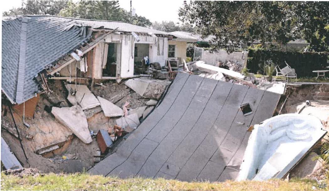
Figure 5.11 – Sinkhole Collapse of a House
