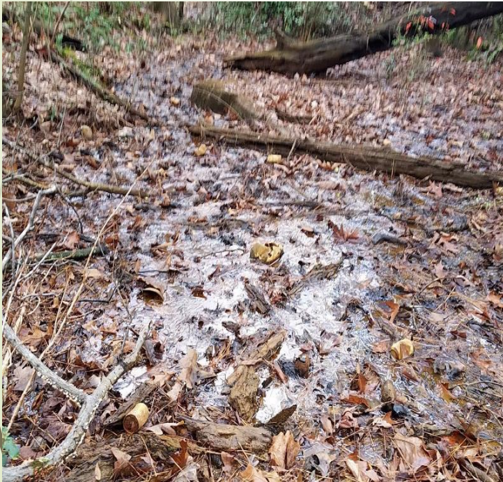
Seepage at Toe
