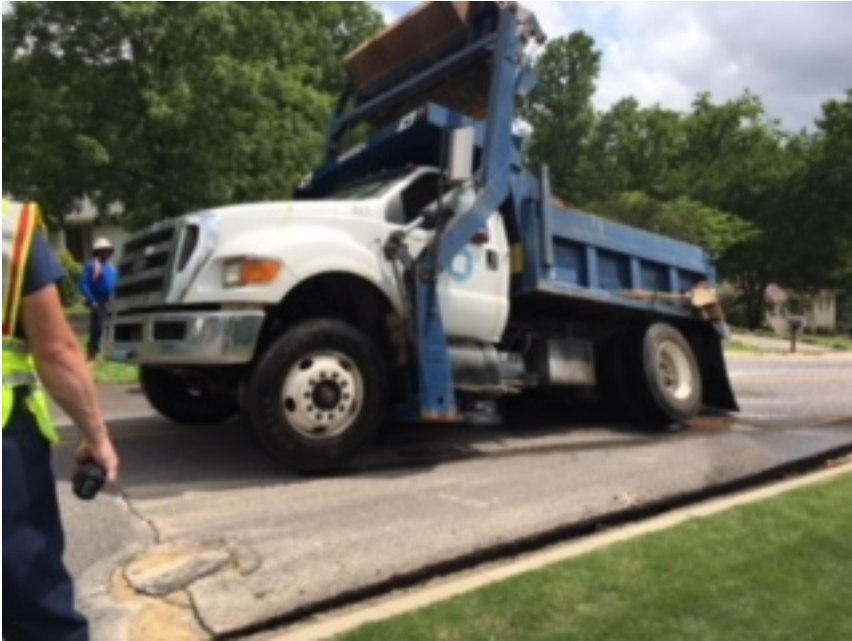
1720 Vestaview Lane, BWWB main burst, 6/1/18
