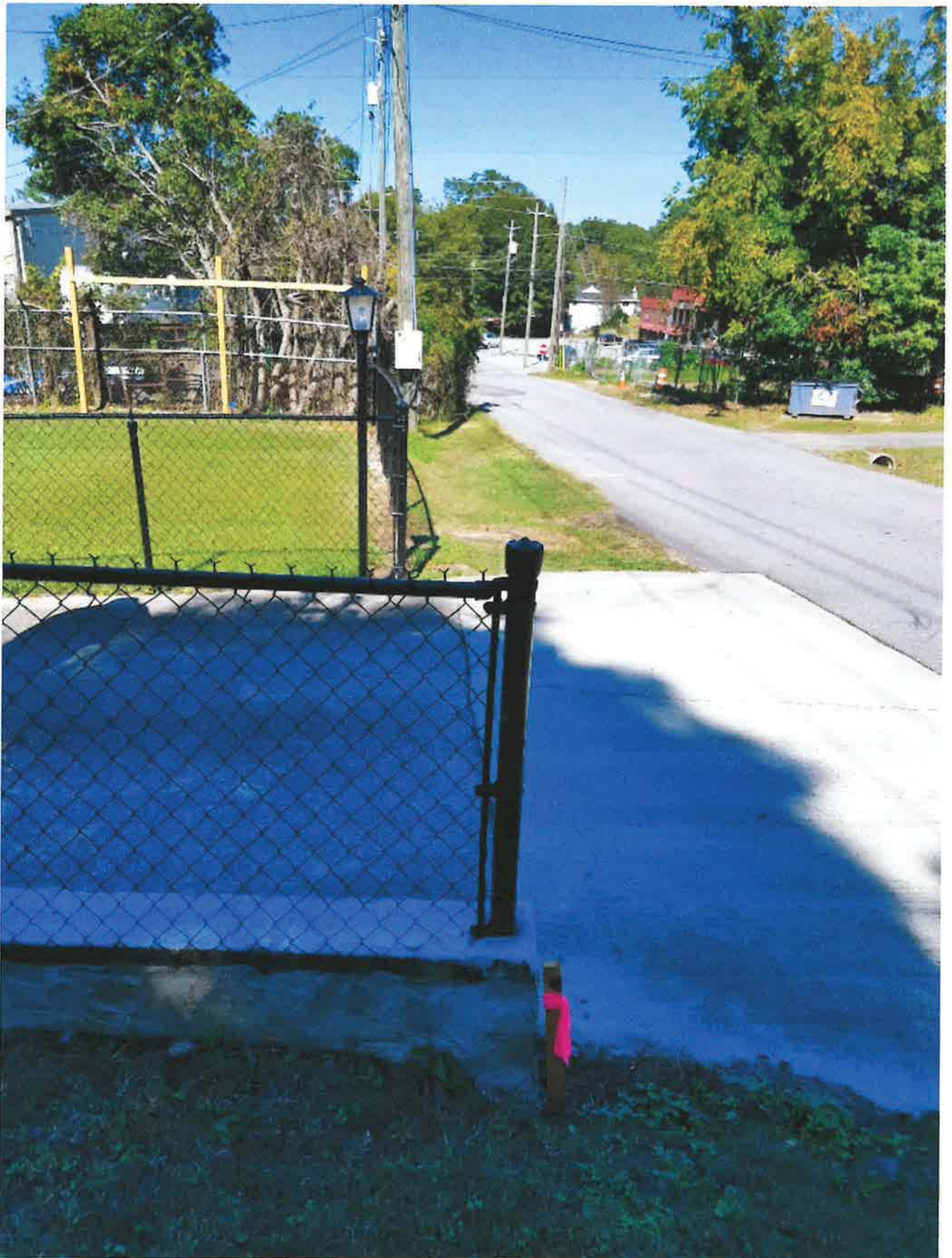
View driving down White Oak Drive NOT blocking Right of way OR Power lines
