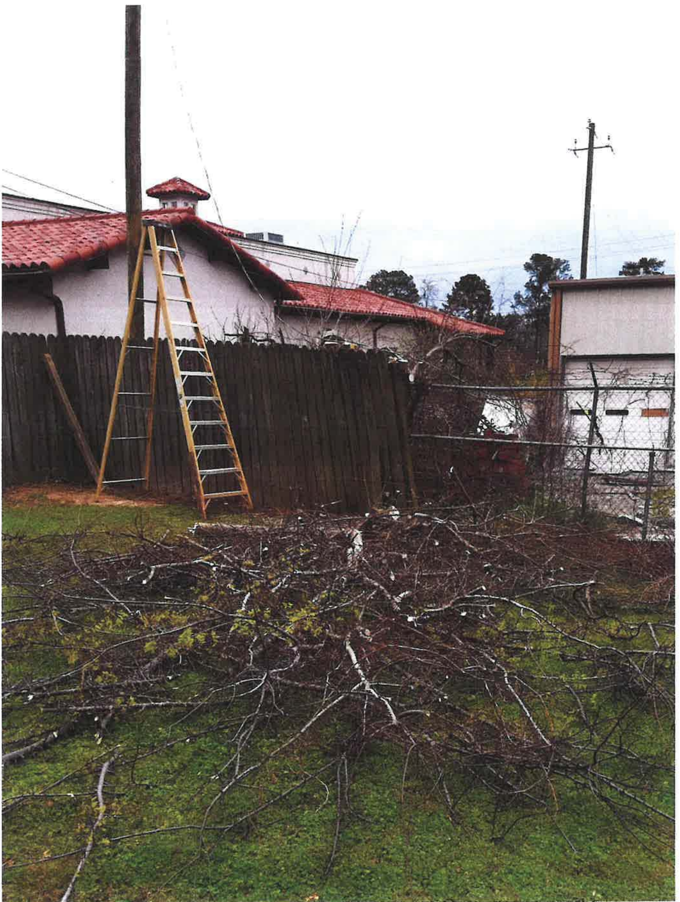
Previous 8ft falling down due to age and trees growing between chain link fences.
