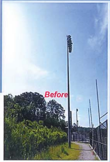
AT&T Liberty Park South (ID# 12778284) Vestavia Hills, Alabama 125-foot Light Pole Tower As viewed from North
