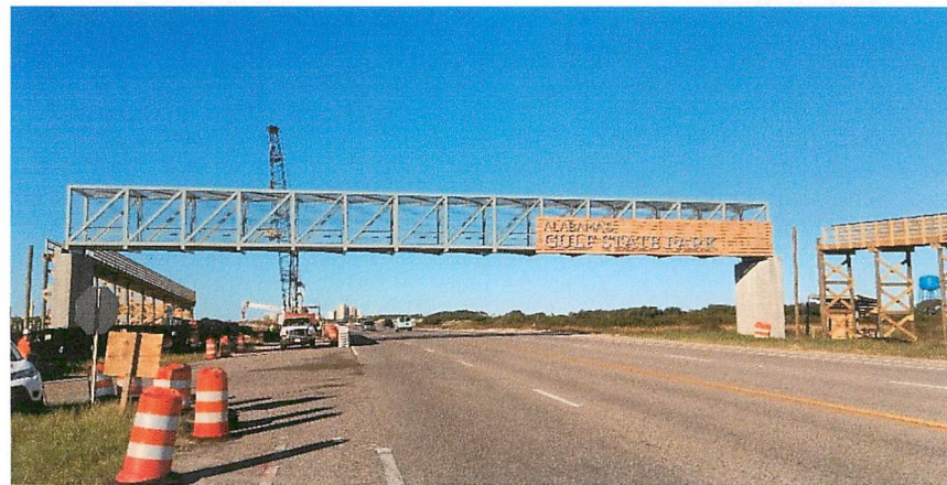
Figure 2: Front Beach Rd, Gulf Shores, AL; Contractor: Banner Industrial Construction, Inc.; Truss Supplier: Qualico Steel
