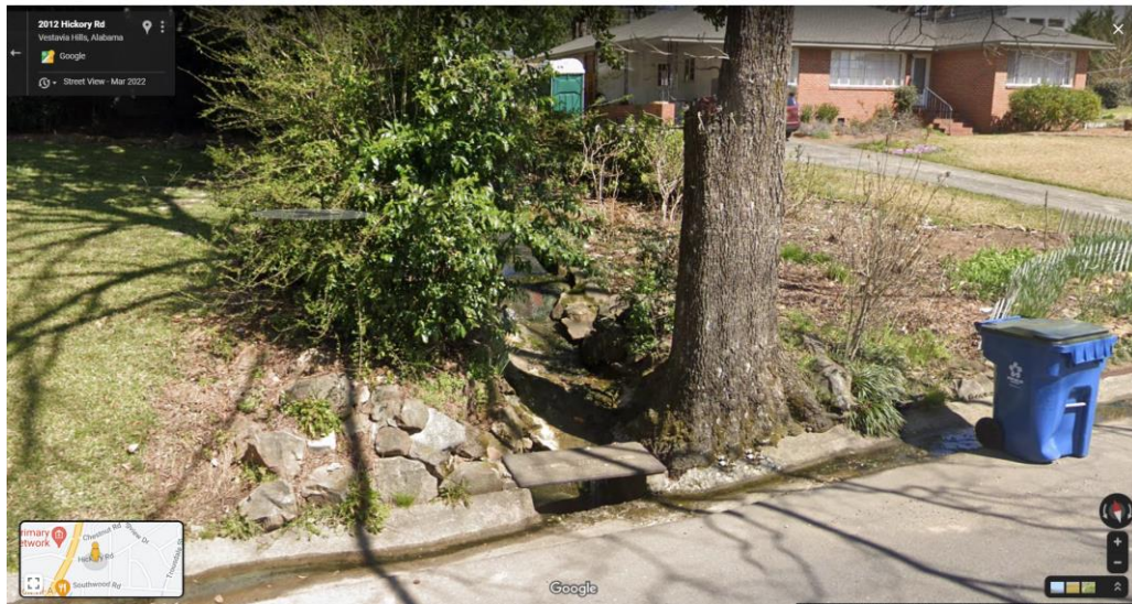
Figure 5 – Beneath this flume is the 18-inch concrete pipe. Both the flume and the pipe discharge into the back side of the inlet shown above. Earth Imagery dated March 2022.
